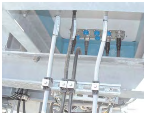
Kabelanschlüsse / Cable connections
